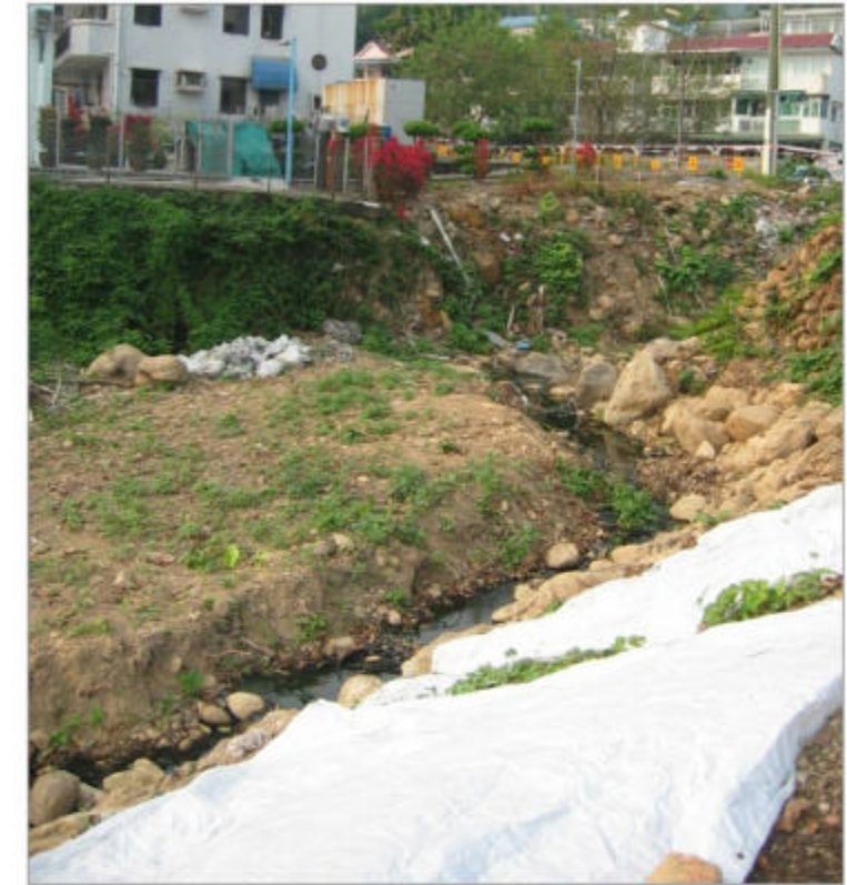
The lower course of stream S3 was highly disturbed by the construction activities of the village area.
