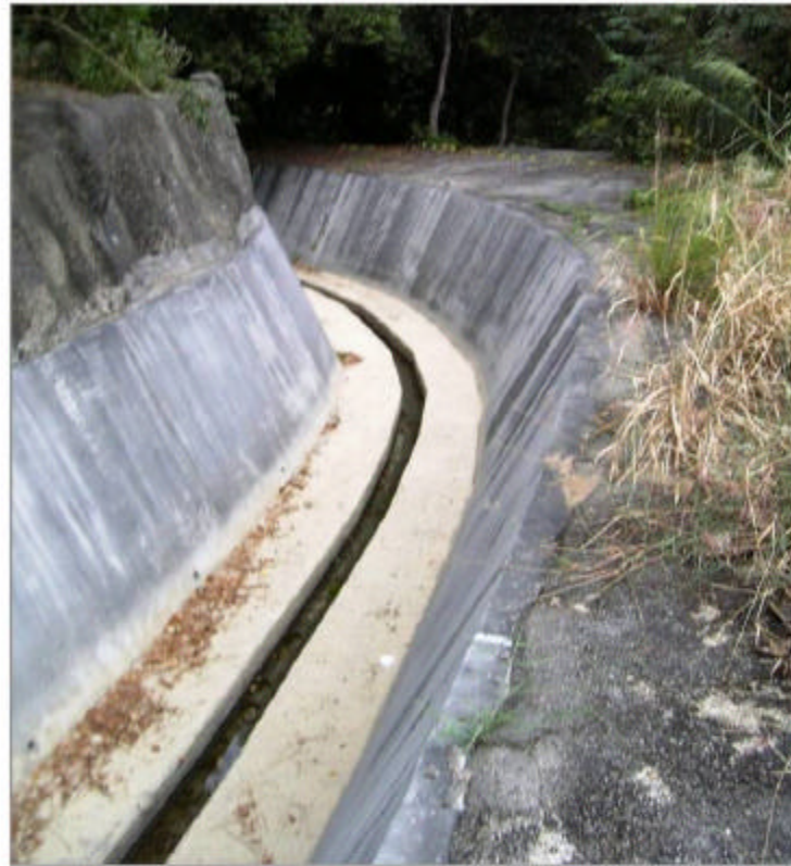
Drainage channel S2 was found at the fringe of Pat Sin Leng Country Park.
